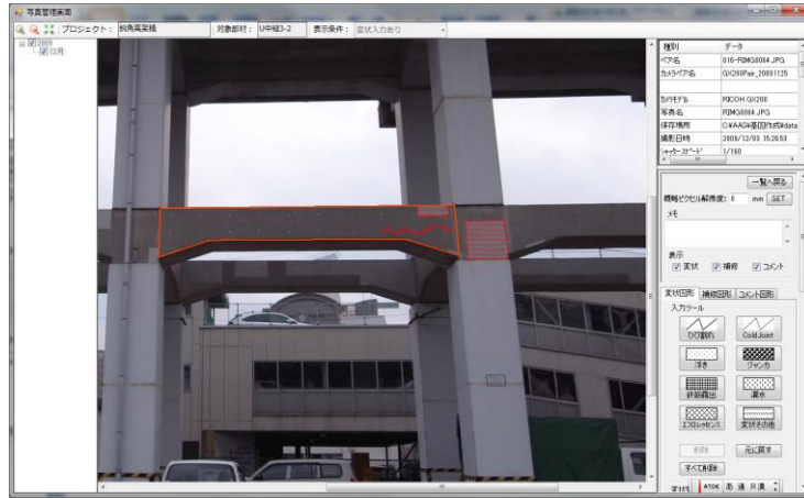
Fig. 10. Tracing of records of damages and repairs on the photo
